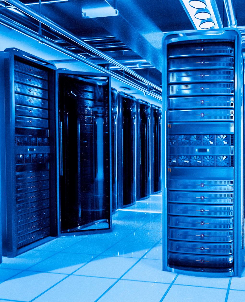
NETWORK SERVERS RACKS. PHOTOGRAPH BY XH4D/ISTOCK
