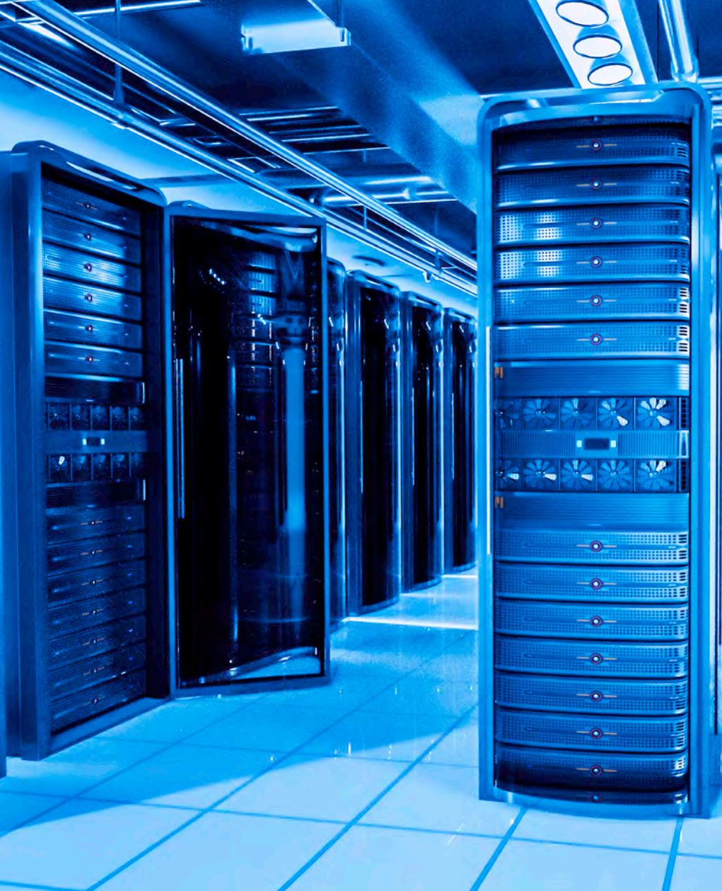
NETWORK SERVERS RACKS. PHOTOGRAPH BY XH4D/ISTOCK
